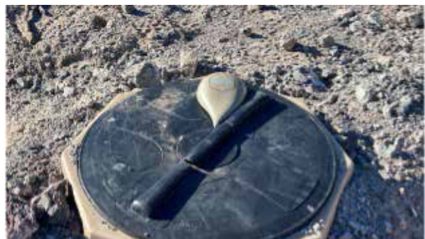
Track Tag, LLC. Water level transducer and Bluetooth transmitter, SL13 Hawkeye tank #1
