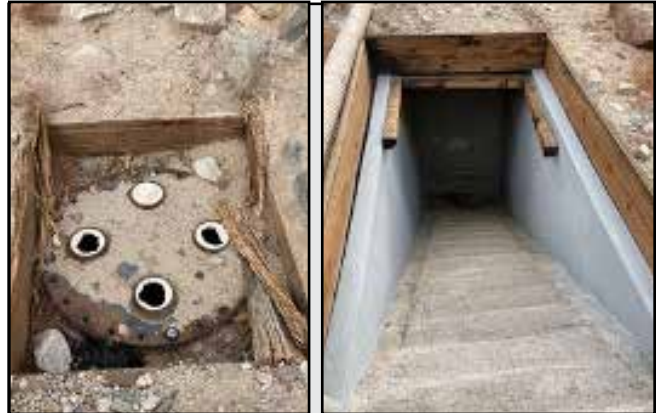
Preliminary visit showing vandalism and an empty tank. Photos above courtesy Andrew Pontious
