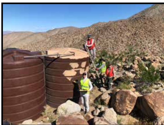
New tanks at Pinyon Wash getting a coat of paint to protect from the sun's damaging ultraviolet rays and to camouflage.
