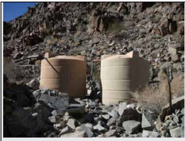
Tanks installed in 1979 as they appeared in 2004
